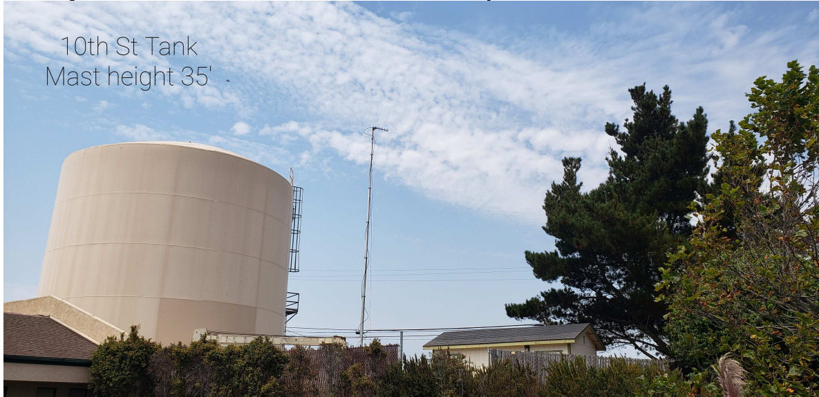
Figure 16 – 10th Street Tank Repeater Site
